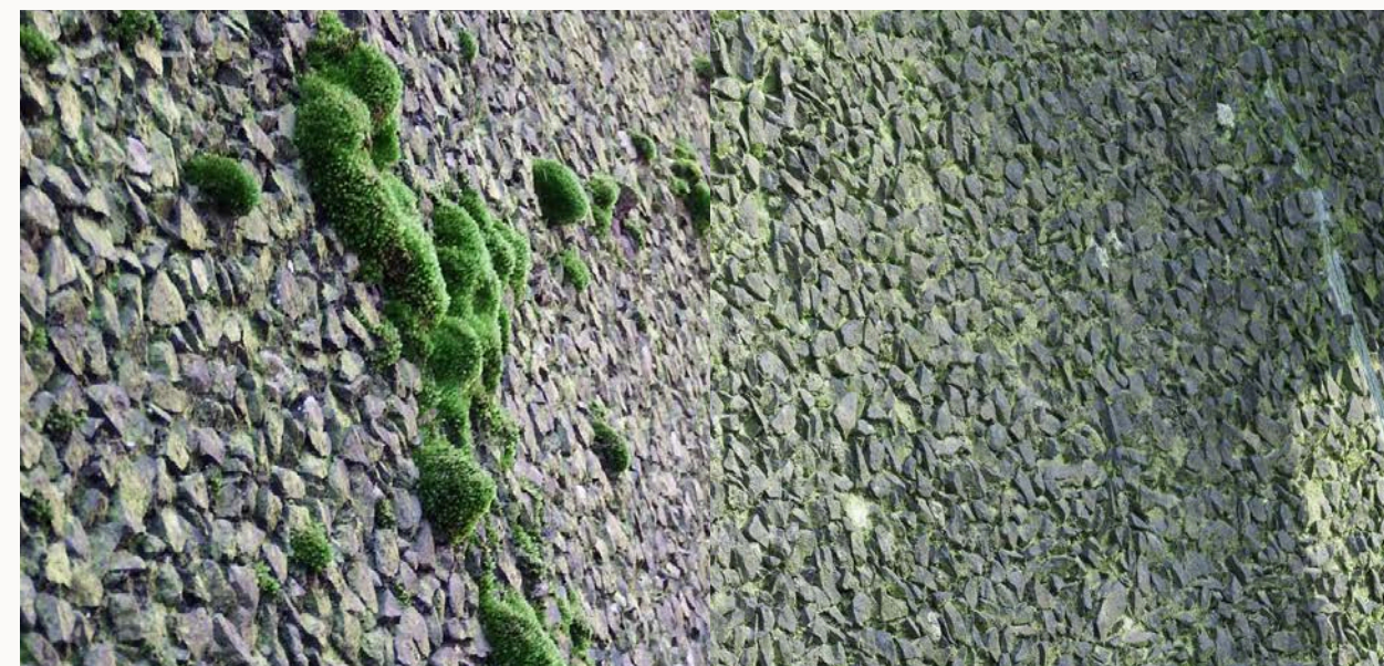
OBS. 05 — GROWTH BETWEEN THE CRACKS
