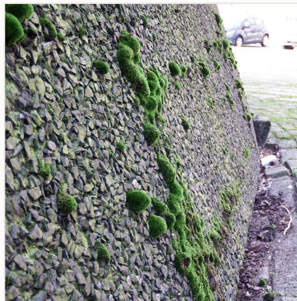
Fig. 5.15 — Moss growing on rough concrete surface with imbedded rocks.
