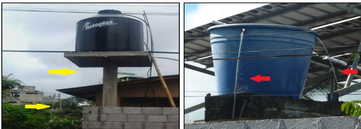
Figure 4.6-Pictures of typical spilling tanks in Puerto Ayora.
