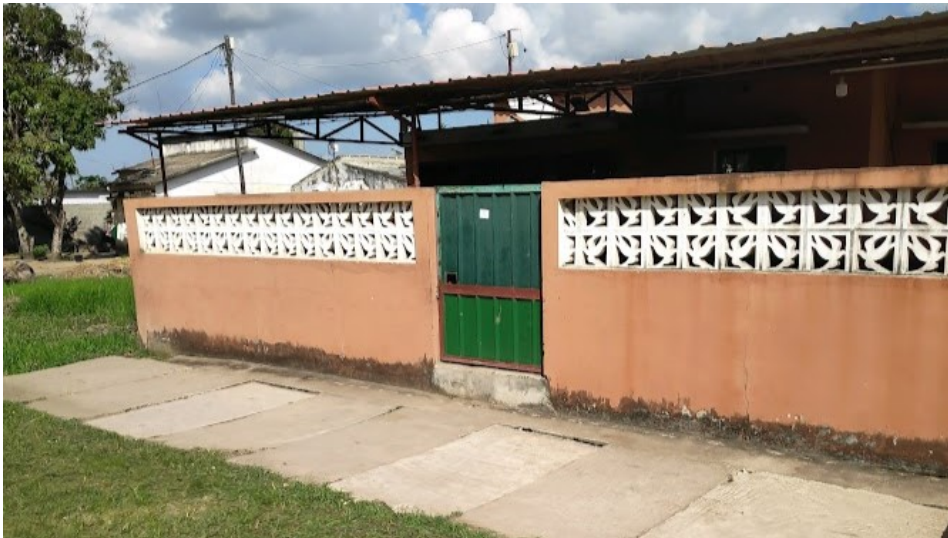
Figure 2.2: Raised doorstep as a flood mitigation measure on a household scale in Manga, Beira (picture by author)
