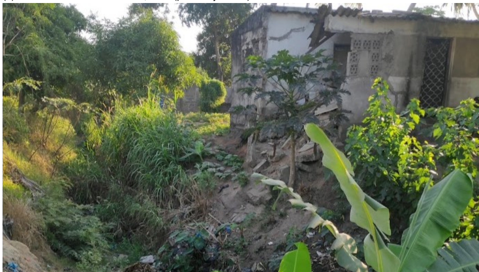
(b) Erosion of a canal side wall, causing the collapse of a house next to a bridge in Manga, Beira (picture by author)
