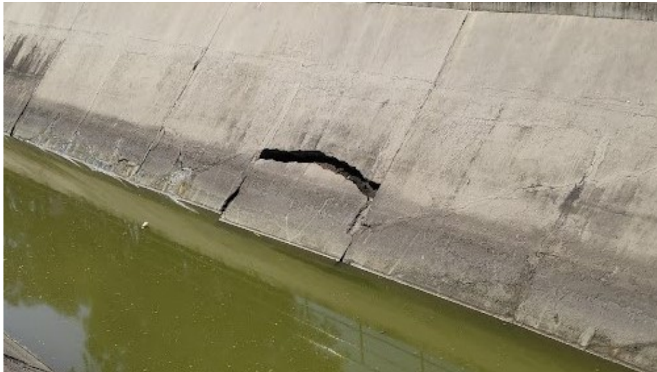
(a) A broken side wall in Munhava, Beira (picture by author)
