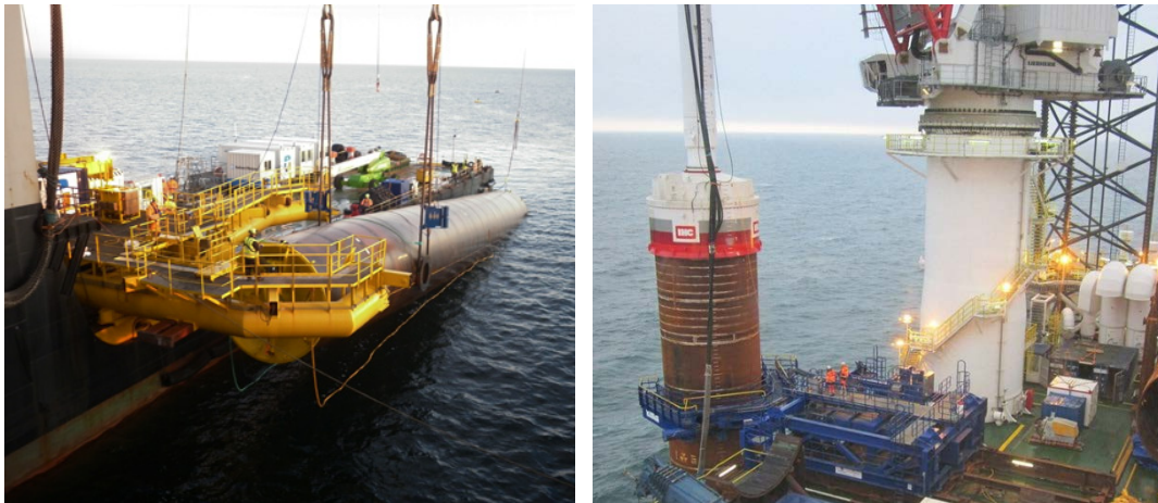
Figure 10 Lifting the pile (left) and hammering the pile down through the alignment tool (right) [9]
