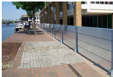
Figure 3.22: Practical example of a local flood wall, which is a form of dry proofing (source: Flood Control International, 2020)
