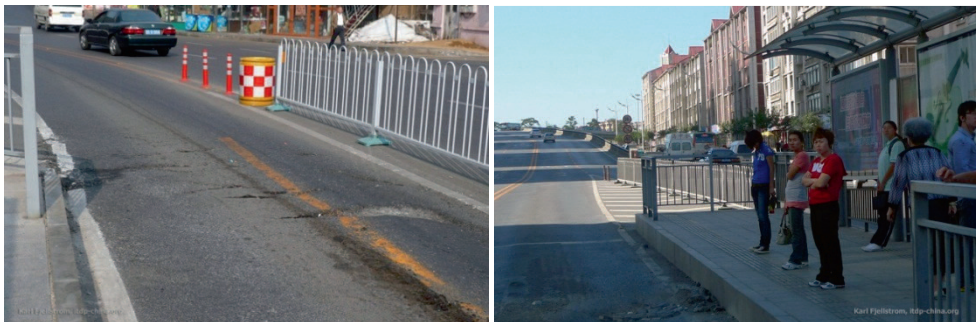
Note: BRT lanes lack maintenance and the road surface conditions are poor.
