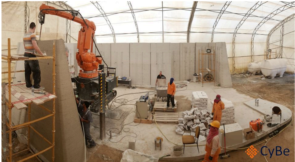
Figure 32 Cybe 3D concrete printing robot on the construction site in Dubai © Cybe
