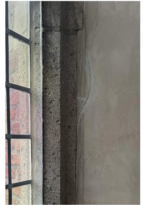
OUTSIDE AIR INFILTRATION THROUGH CRACKS
