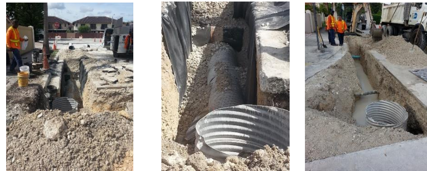
Image 16, 17 & 18. Drainage system of inlets and pipes in Hialeah. Source: Michael Sukop.
