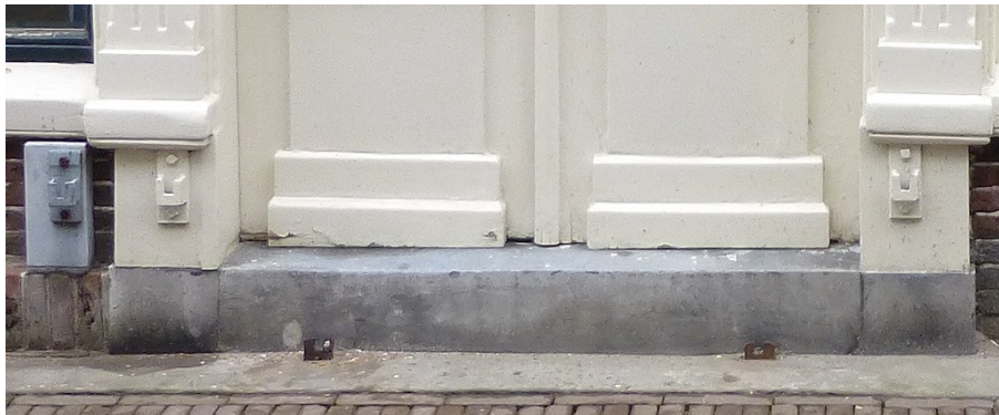
Figure A.2: Dordrecht: fixtures for temporary sealing of door openings with stop logs in houses along the Voorstraat in Dordrecht, March 2013
