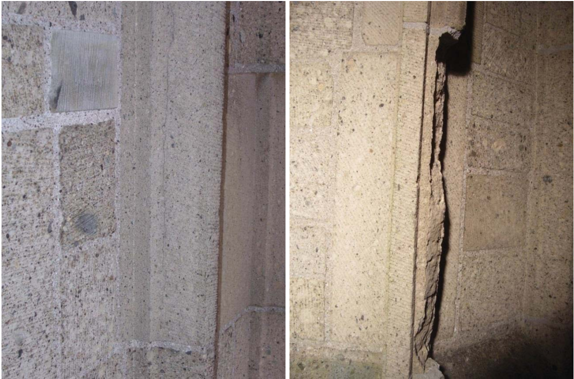
Fig. 1. Typical longitudinal cracking (left) and final damage in mullions of Ettringen tuff at the tower of Eusebius' church in Arnhem, The Netherlands (pictures T.G. Nijland, 2009).
