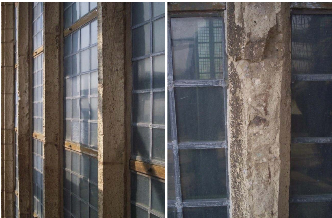
Fig. 2. Typical longitudinal cracking (left) and final damage in mullions of Weibern tuff at the nave of St. Peter's church in Leiden, The Netherlands (pictures T.G. Nijland, 2005).
