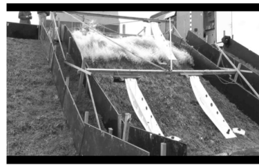
(b) Separation from the landside slope
