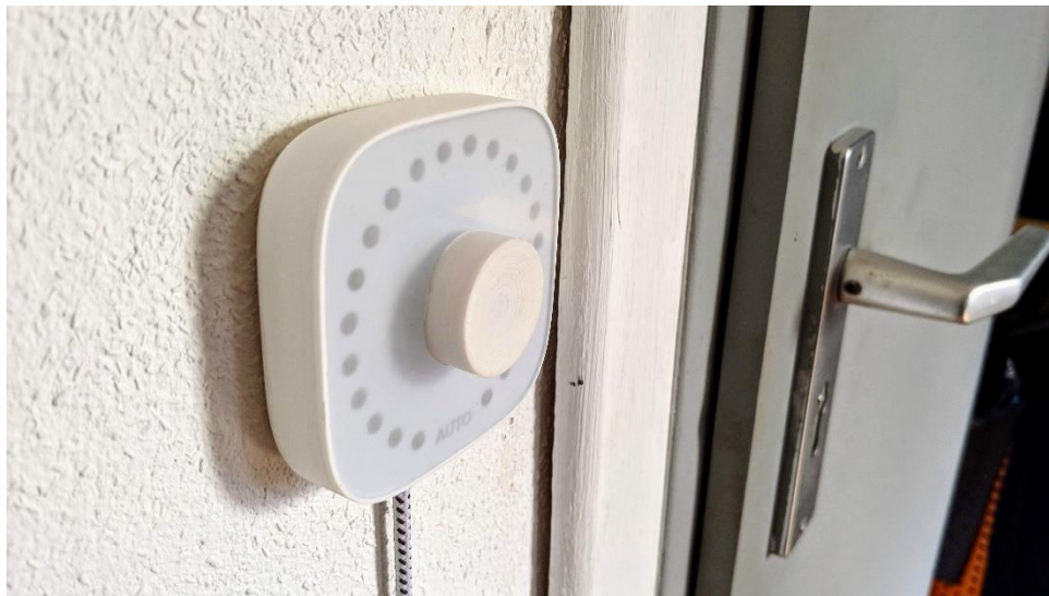
Figure 50: The dimmer placed on a wall next to a door, where it's expected.
