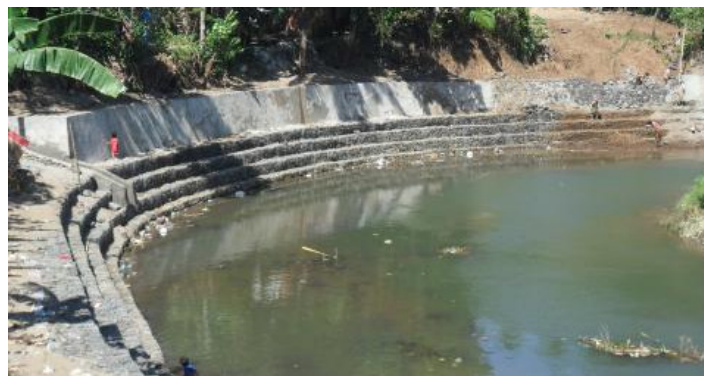
Figure 12: Revetment improvement in Tikale watershed
