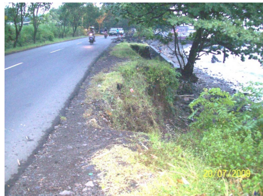
Figure 9: Erosion along the road
