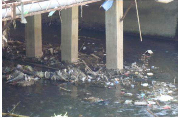
Figure 9: Garbage got caught behind bridge pillars
