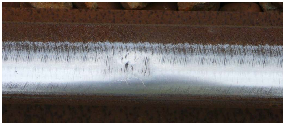
Fig. 1.10 Branching micro-cracks beneath a ground squat at the rail surface
