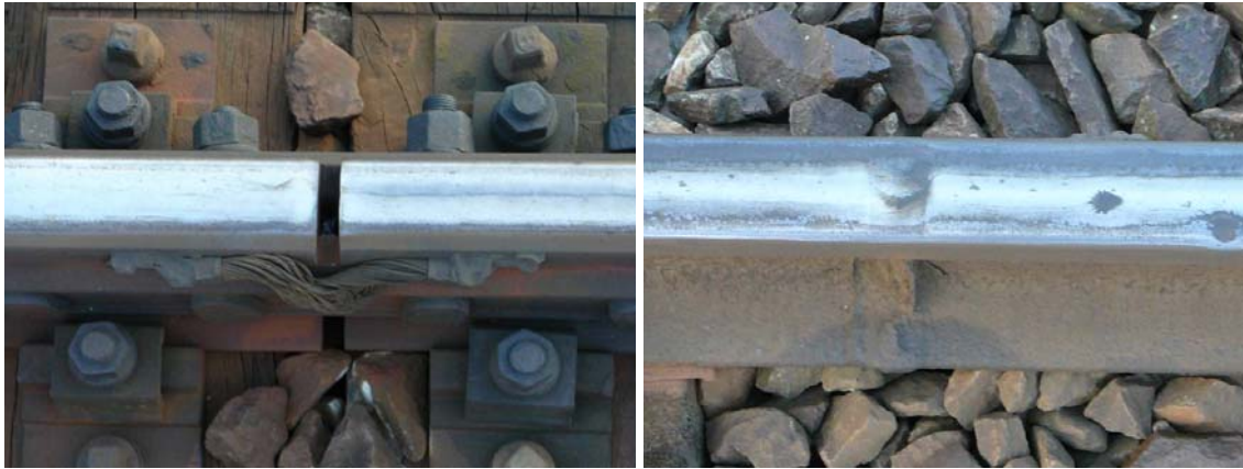
Fig. 1.12 Insulated rail joint with wide gap (left) and rail weld (right)
