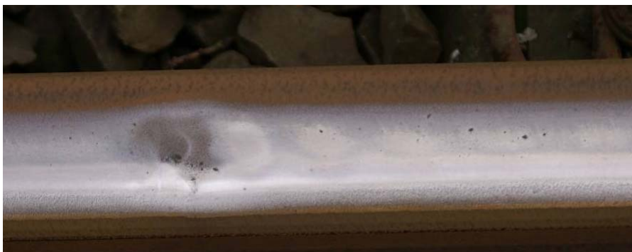
Fig. 4.7 Rail corrugation generated by a squat rail surface irregularity, initiated at a flash butt weld
