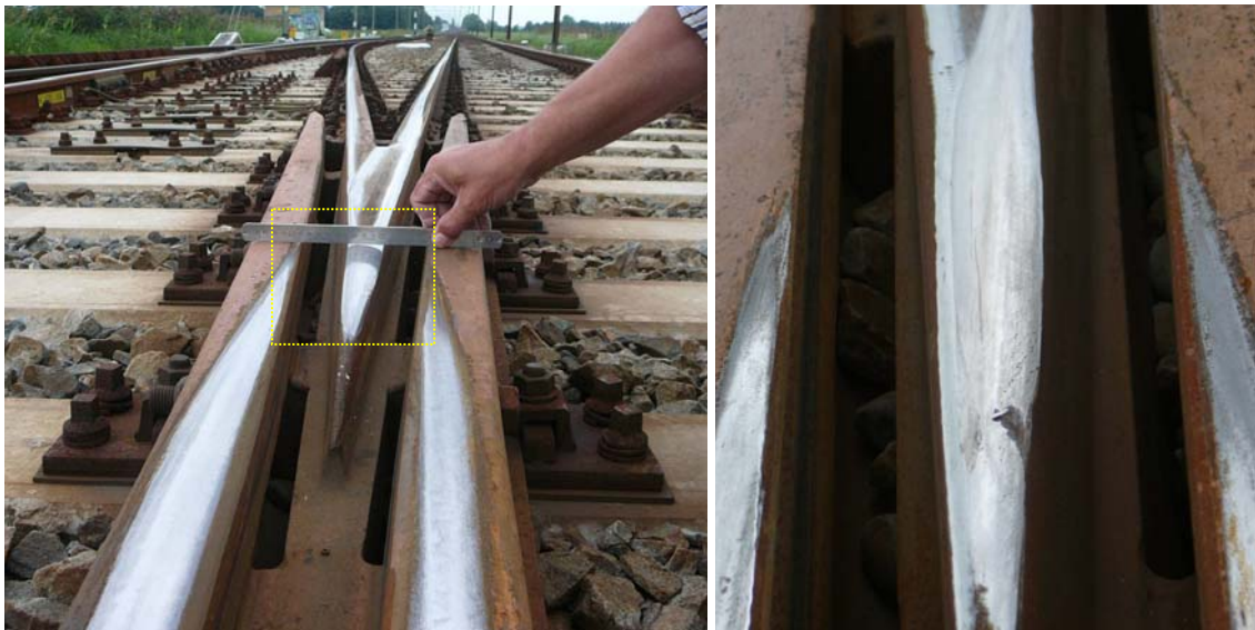
Fig. 1.14 Switch (left); RCF damage at the transition to the nose (right, zoom-in)
