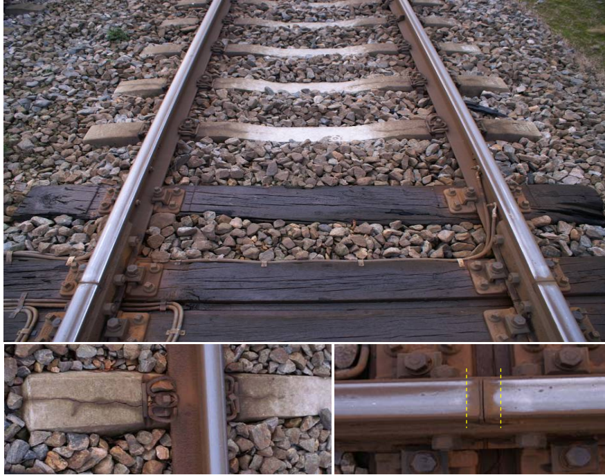
Fig. 2.2 Insulated rail joints with transient double point-contact (zoom-in, right: indicator is the interrupted running band on the railhead) and severe track damage (zoom-in, left: broken sleepers until 3 m after the joints)
