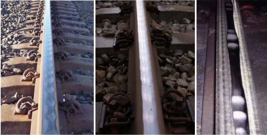
Fig. 1.11 Rail corrugation or rutting (centre)
