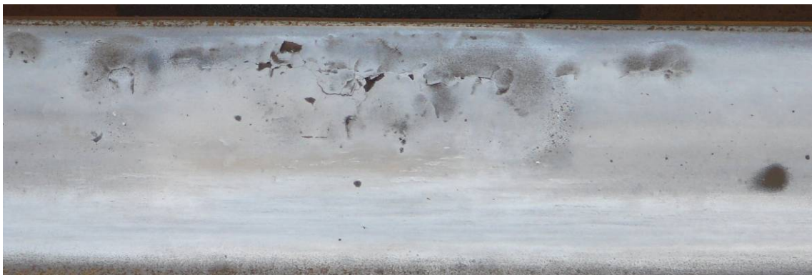
Fig. 1.15 Branching and propagating micro-cracks in the railhead, emerging from internal material defects (squat-like defects)
