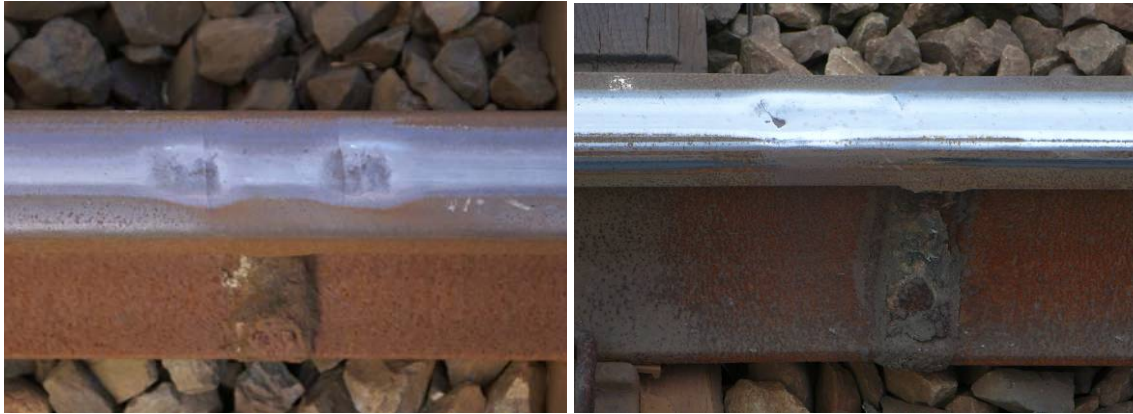
Fig. 4.8 Squat initiation on thermite rail welds or in the HAZ (right: accompanied by crack initiation)
