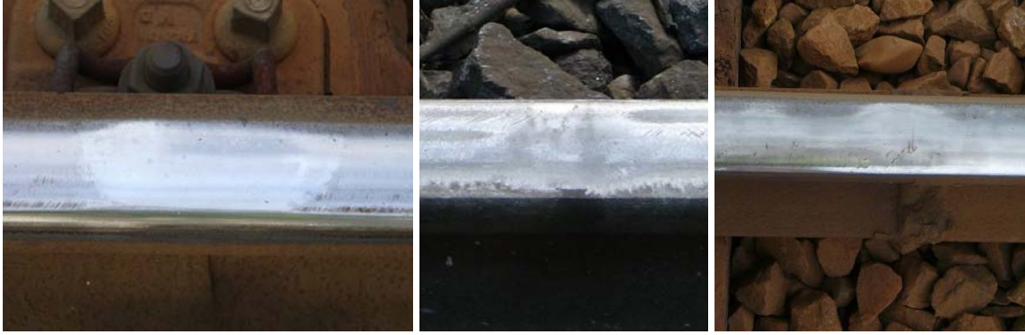
Fig. 4.6 Deteriorating geometry resulting from non-uniform shakedown and work hardening along a rail weld in the HAZ (left: flash butt weld; centre, right: thermite weld)
