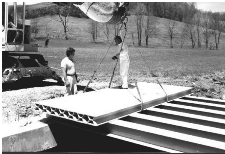
Figure 5.5: Installation of Laurel Lick Bridge, West Virginia, the United States, 1997 (Creative Pultrusions Inc., Alum Bank, PA.)
