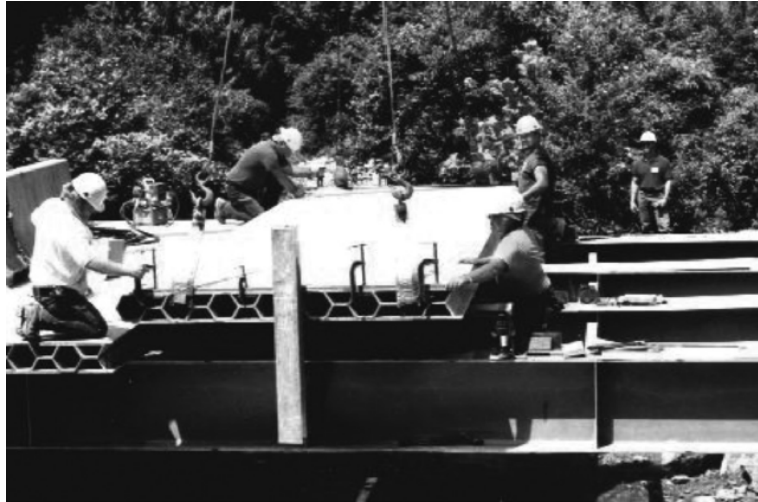
Figure 5.4: Wickwire Run Bridge during installation, Taylor County, West Virginia, 1997 (Creative Pultrusions Inc., Alum Bank, PA.)
