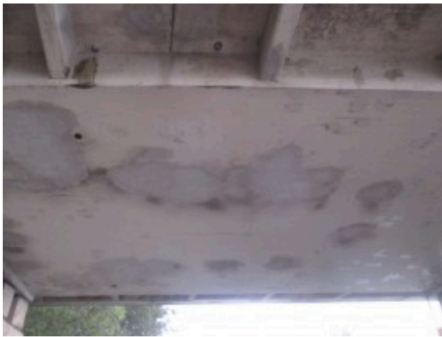
Fig. 6. Damage to the bottom of the reinforced concrete slab.
