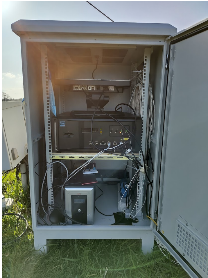
Figure 4.6: The inside of the data acquisition cabinet
