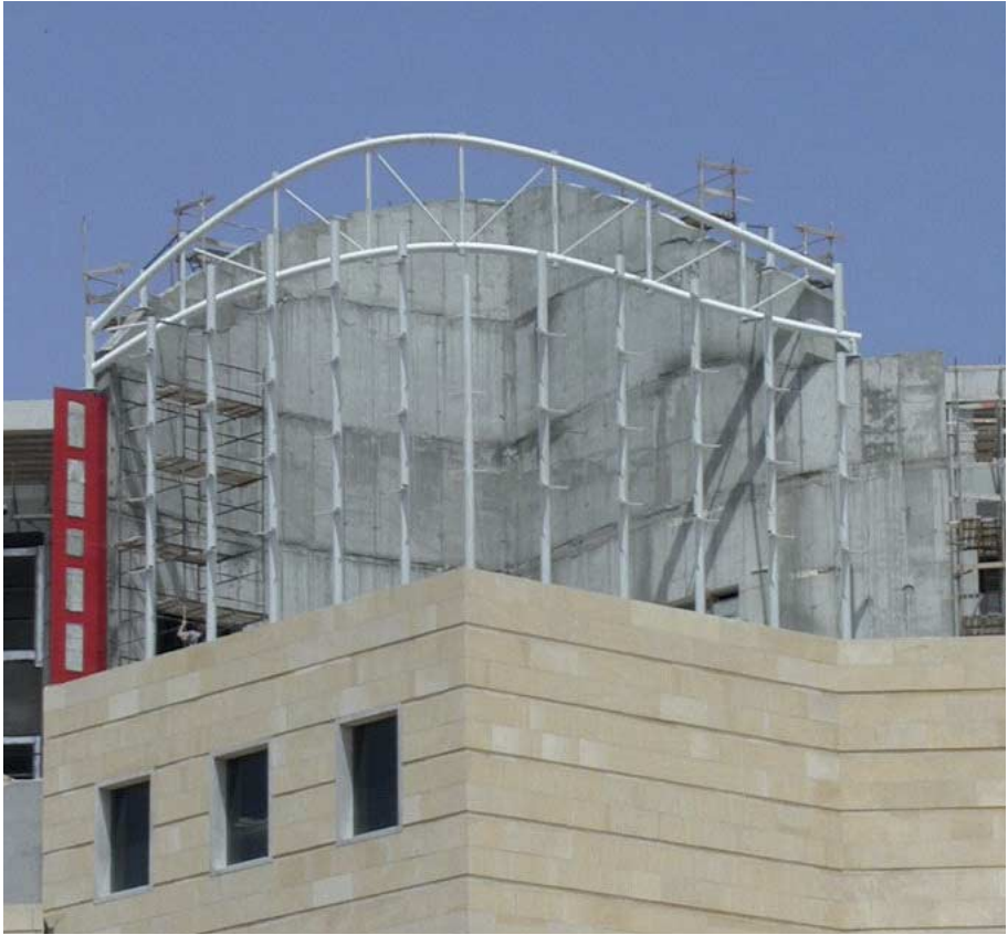
FIG. 81 Building site in Tel Aviv zoomed in on 'The Library' with the truss and columns already installed.
