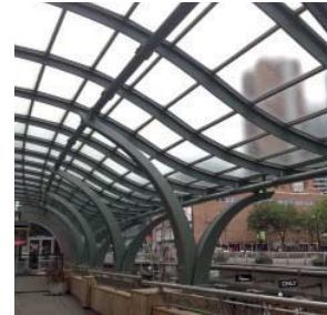
FIG. 143 Curved triangular beam in a canopy of the 'koopgoot' in Rotterdam [NL]. Architect: Architecten Cie
