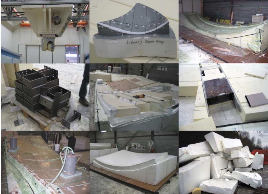
FIG. 76 Milling machine at Marin, scale model of upper wing of 'The Library' and production of the roof segments at Holland Composites. Vacuum injection of the top layer on foam block milled by Marin. Insert to be placed in the GRP sandwich roofs in order to make a connection between the roofs and the columns. Placement of foam blocks and glass fiber mats, which will become stringers. Vacuum injection of the bottom layer. Final result, in this case an early prototype. Discarded foam moulds.
