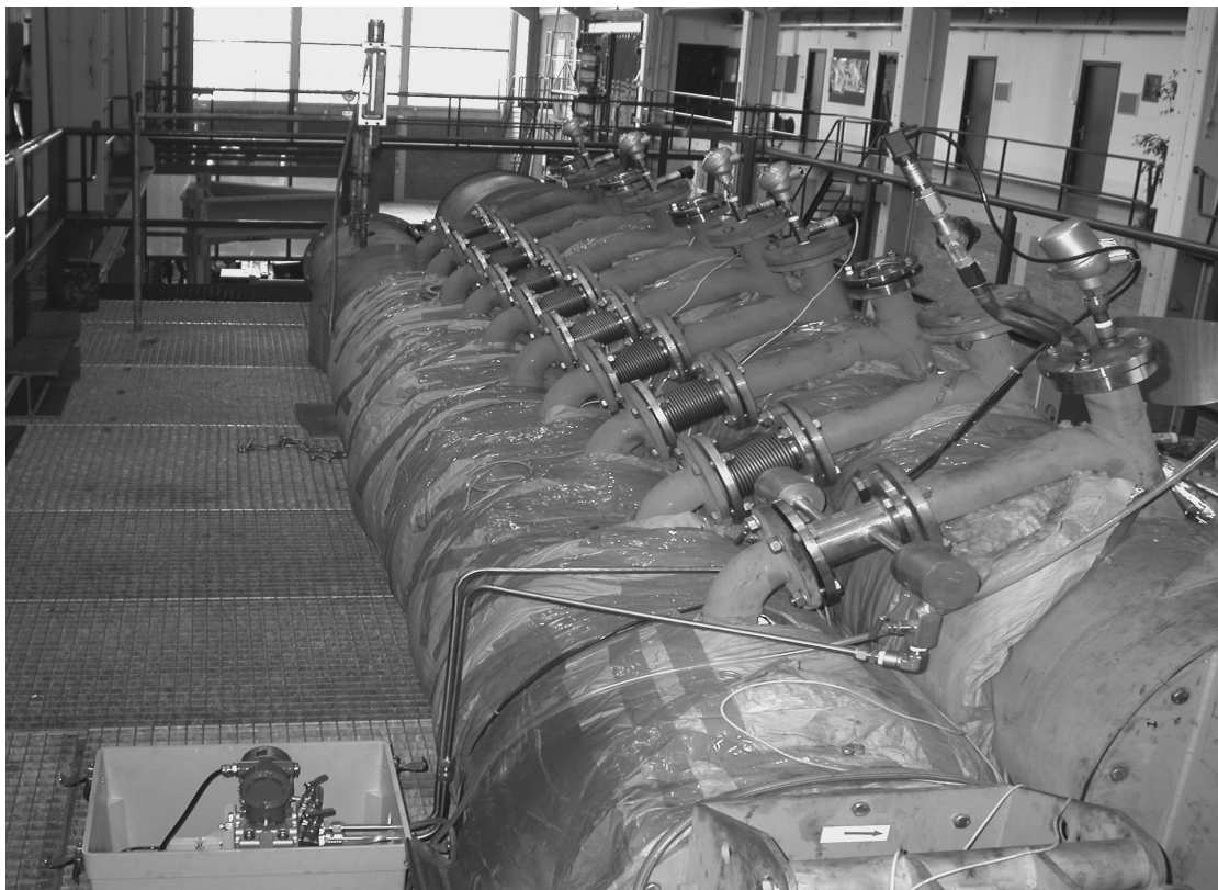
Fig.7.7: The two screw conveyors of the prototype, partly wrapped in insulation material. The vapour bridges were equipped with pressure transmitters and thermocouples.
