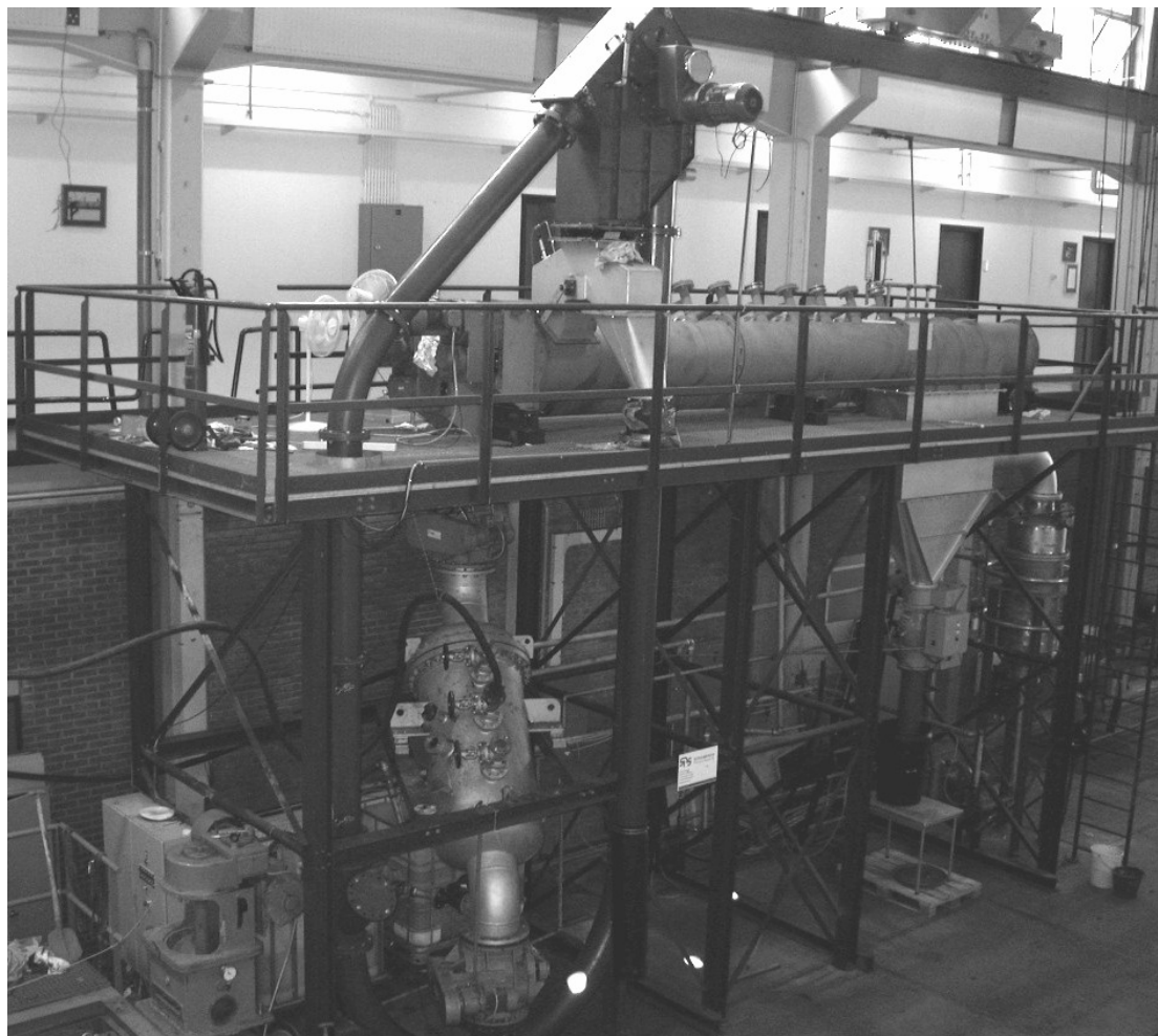
Figure 7.10: The Delta dryer prototype without insulation. The installation has a footprint of 10m x 3m, and height of 8m.
