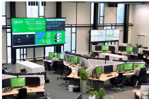
Figure 40: OCCR control room (source [24])
