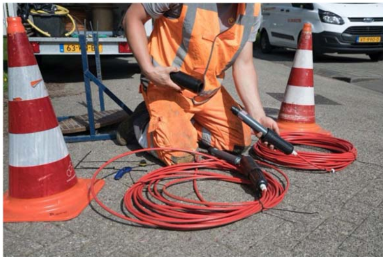
Figure 6.15 Connecting cable segments using an optical connector for DTS measurements. Source: courtesy Remy Schilperoort (Partners4UrbanWater).
