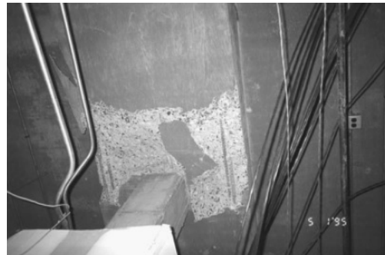
Fig.12 Damaged connection between beam and column (Osteraas, 2006)
