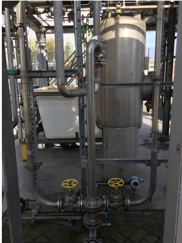
Figure B.9: Front view of the riser base. Only the middle riser (ID = 44 mm) has been used.
