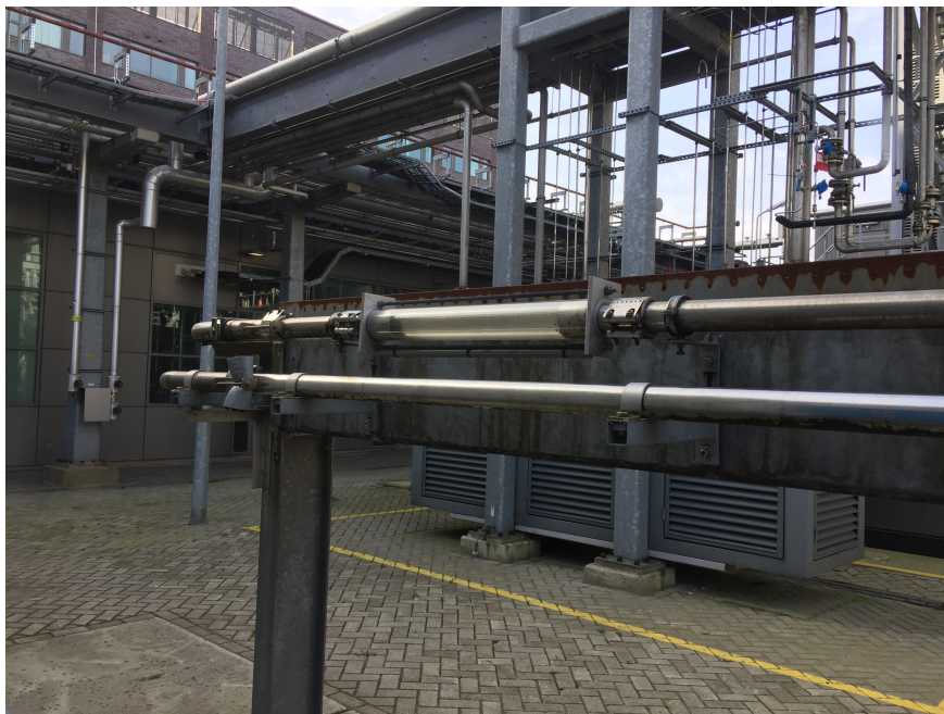
Figure B.3: The inspection glass on the horizontal flowline.
