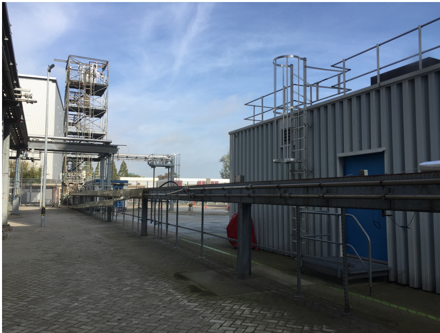
Figure B.8: Photo of the SSL with the vertical riser (installation platform on the left) and the horizontal flowline (all the way to the right).
