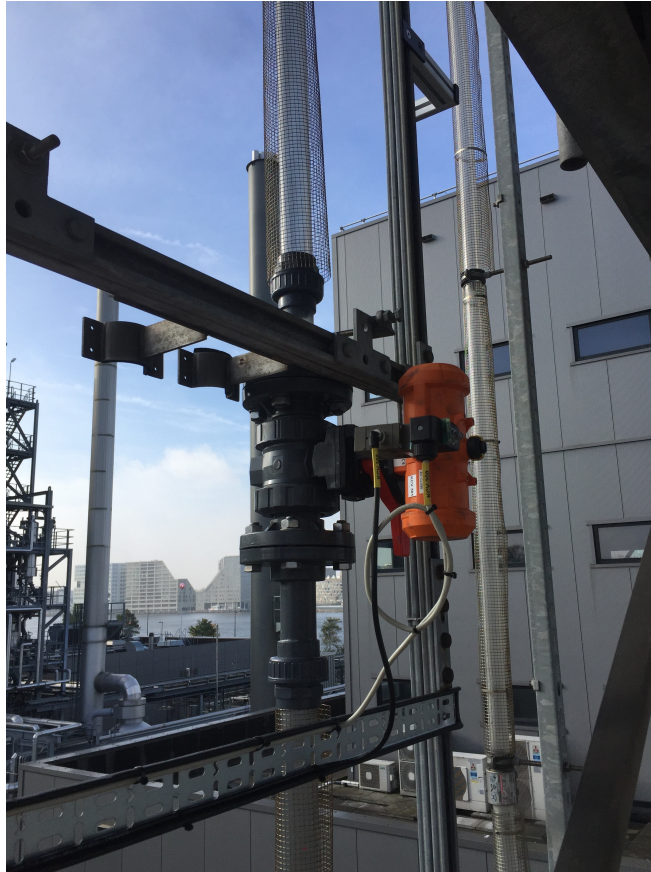
Figure B.7: The quick closing valve installed on the riser (KCV-300).
