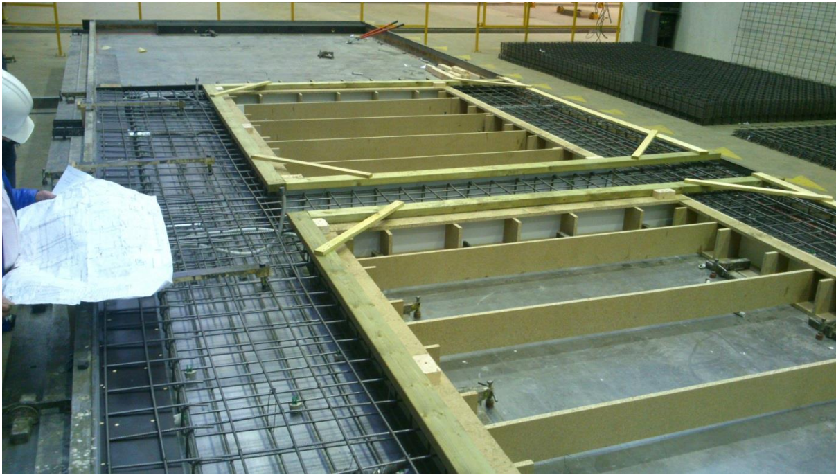
FIGURE 16: A MOLD ON ONE OF THE TABLES, READY FOR THE CONCRETE POURING
