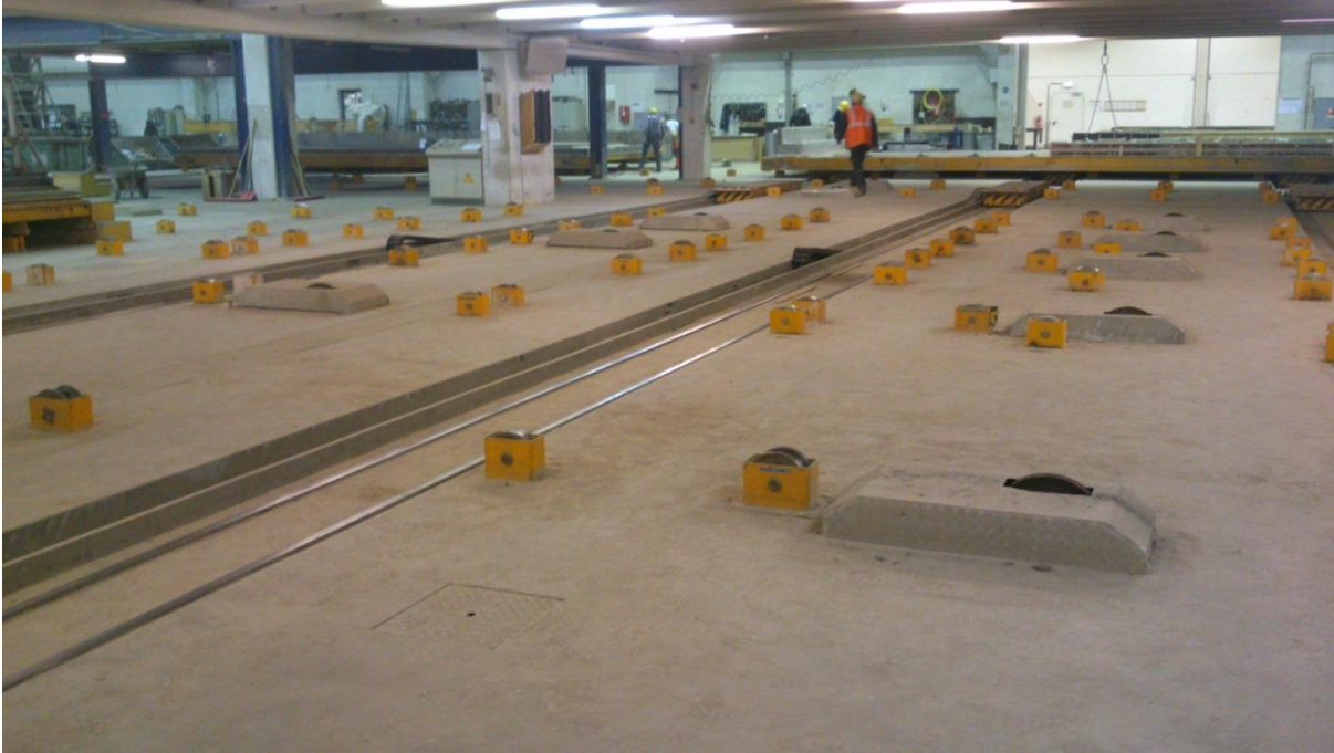
FIGURE 15: THE ROLLERS AND CARTS THAT MOVE THE TABLES AROUND
