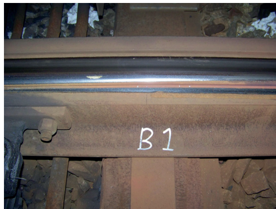
Figure 15. Switch panel of ‘mild’ wearing switch (left switch and stock rail). No wear debris observed. At the gauge face remains of lubrication are present.
