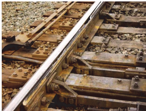
Figure 11: Example of excessively worn and spalled switch rail
