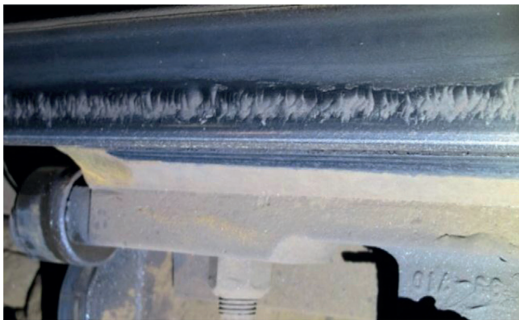
Fig. 3. RCF damaged stock rail.
