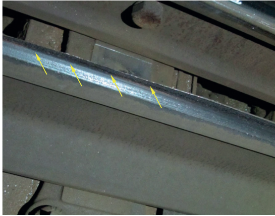
Figure 12. Severely worn switch rail (inspection December 2014).
