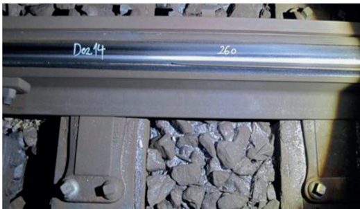
Fig. 2. Severely worn and locally spalled switch blade (wear debris visible at sleepers and in ballast).
