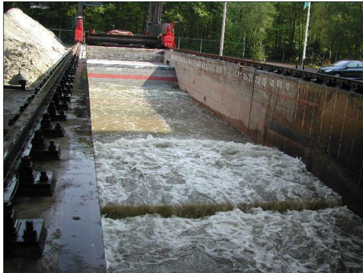
a. Overtopped water on revetment
