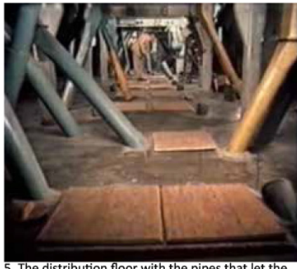
5. The distribution floor with the pipes that let the grain into the silos
