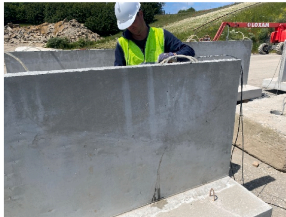
Fig. 4. Supplying the network with water repellent agent; fluid is seen seeping out of the primary crack at the bottom of the wall.
