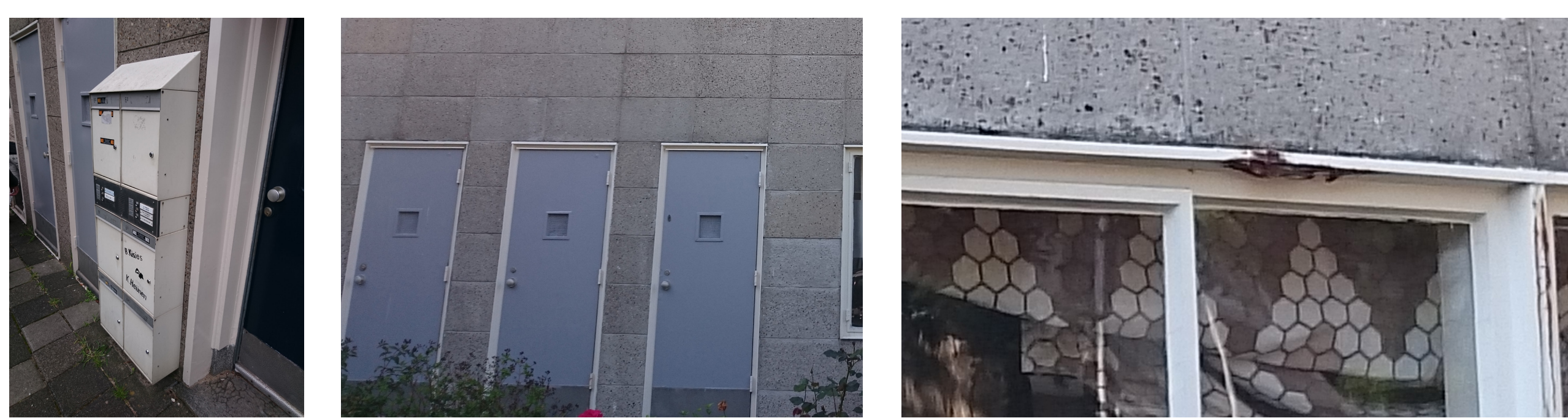
PHOTOS OF EXISTING SITUATION: DECAY & CORROSION
