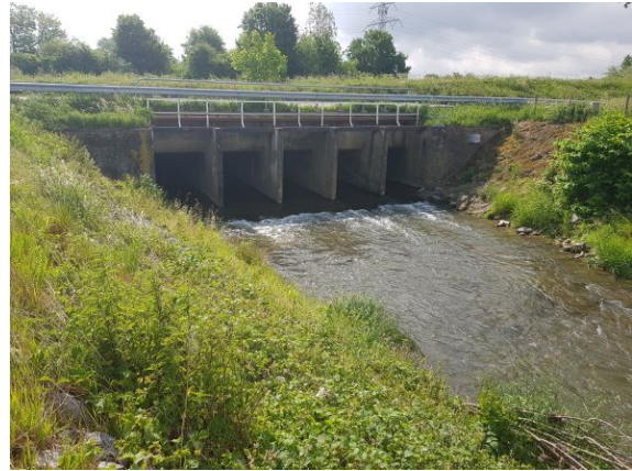
Figure A.5: Outlet of the Geul inverted siphon
