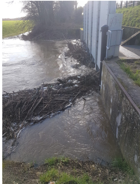
Figure 1.3: Debris at the Geul inverted siphon (3)
