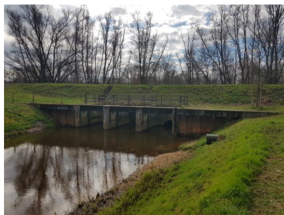
Figure A.2: Outlet of the Tungalroyse beek inverted siphon
