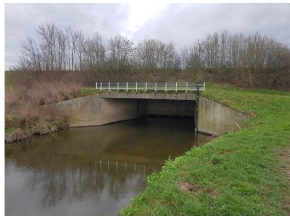
Figure A.9: Outlet of the Tungalroyse beek inverted siphon
