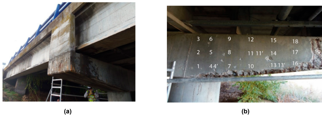
Figure 2.16: Concrete structure studied (a) Condition concrete structure analyzed (b) Points measured on the surface of the beam [18]
