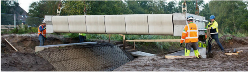
Fig. 6.10 Printed showcase segment for the pedestrian and bicycle bridge (Bos et al. 2019)
