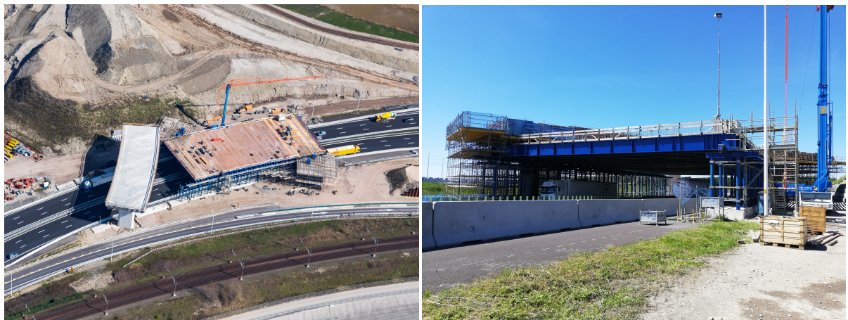
Figure 2.3: Table structure above highway A15, top view (left) and side view (right)
