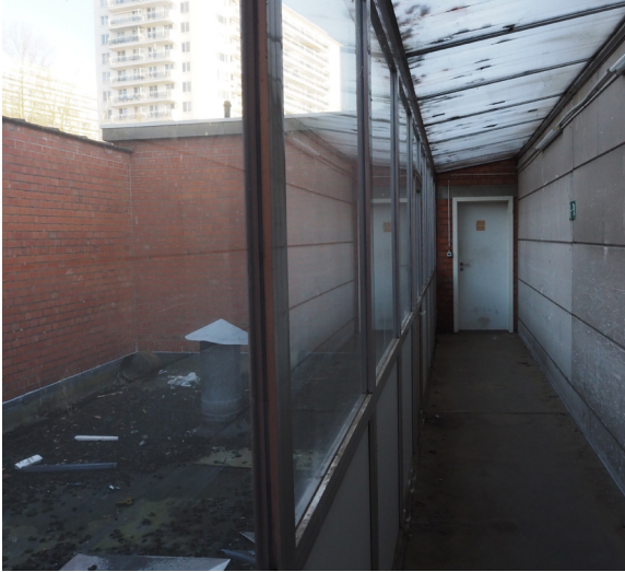
2024, corridor with unaccessible roof
