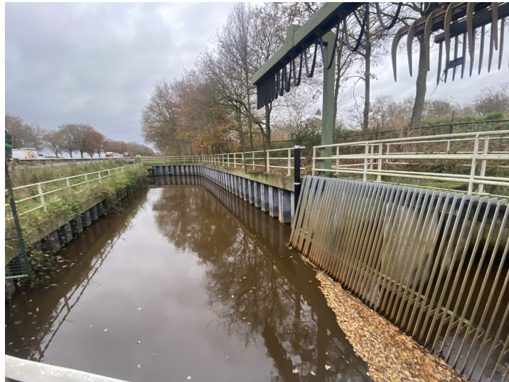
Figure 3.4: Overview of the inverted siphon with trash rack and extraction crane at Uffelsebeek
