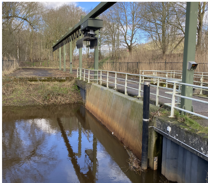
Figure 3.2: Overview of the inverted siphon with trash rack and extraction crane at Tungelroysebeek
