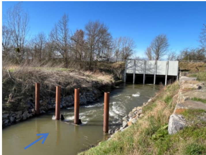
Figure 3.3: Overview of the inverted siphon and interception columns on the upstream side at Bunde
