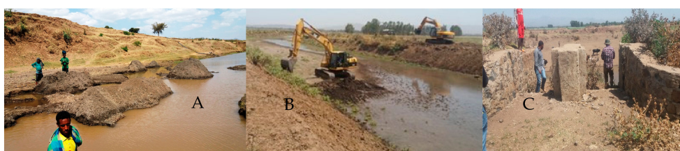
Figure 8. (A) excavated sand accumulation by sand miners in the Middle River reach; (B) river channel enlargement and deepening to increase flow conveyance. The contractor used the material for embankment construction at the Lower reach; (C) flood outlet structure to the farmlands as low height weir (April 2016).
