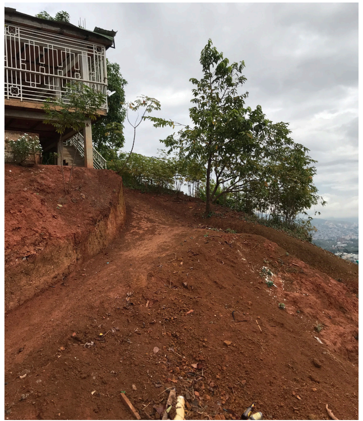
Fig. 66 Evidence of mass movements and terrain instability in the area. Picture by author.
