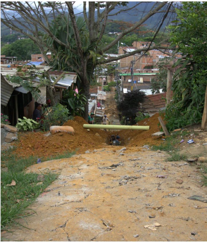
Fig. 68 Ongoing construction of water and sewage infrastructure in areas still lacking basic services. Picture by Gynna Millán.
