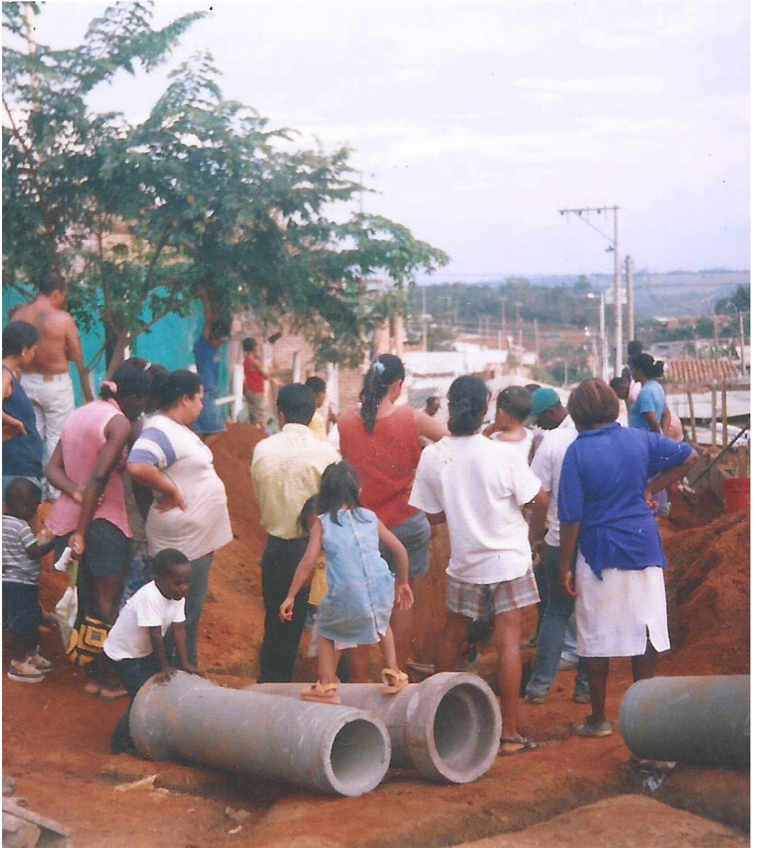
Fig. 49 Community-led installation of sewage system during the early stages of the self-built neighborhood Brisas de las Palmas. Picture by Francy Mina.
