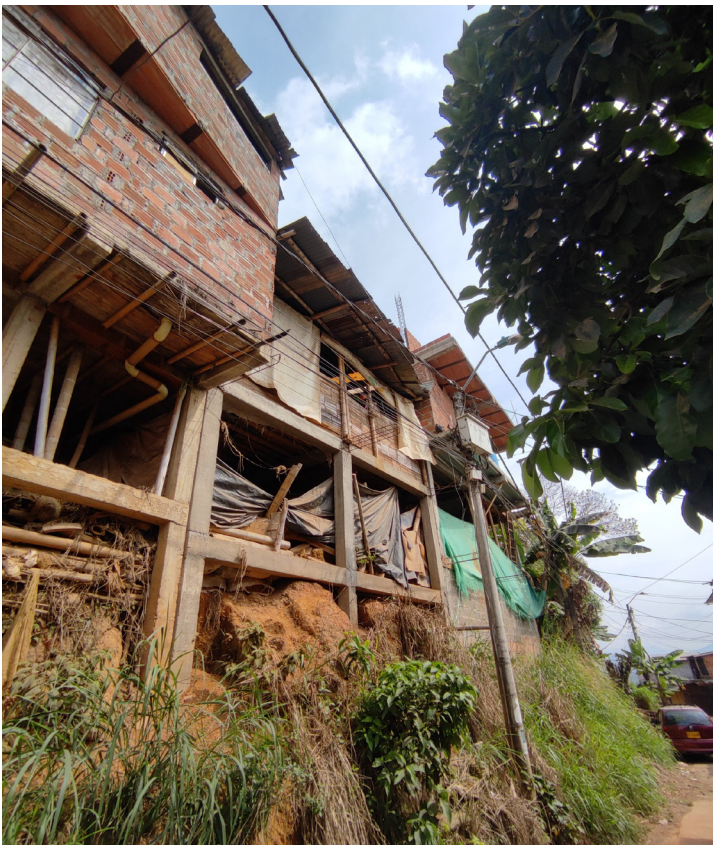
Fig. 65 Exposed structural foundations in homes, highlighting potential danger for residents. Picture by author.
