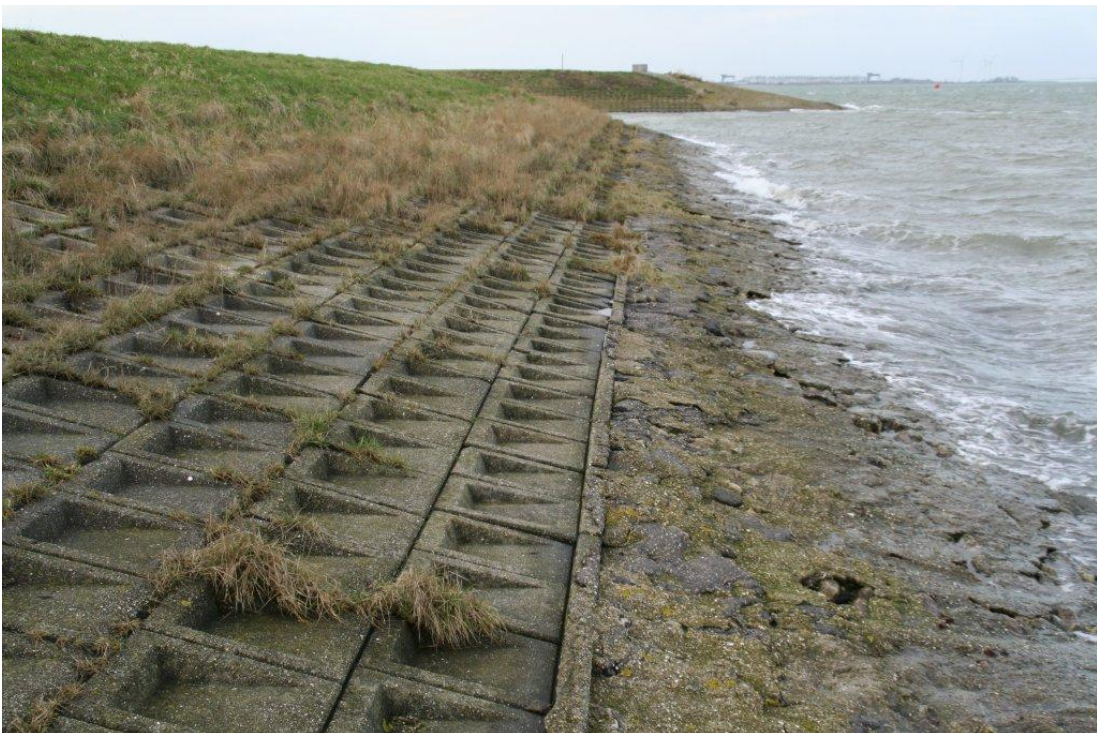
Figure 2.12. Dike near Wilhelmadorp, Zeeland. Design water level 3.5 m +NAP; design wave height 1.1 m.
