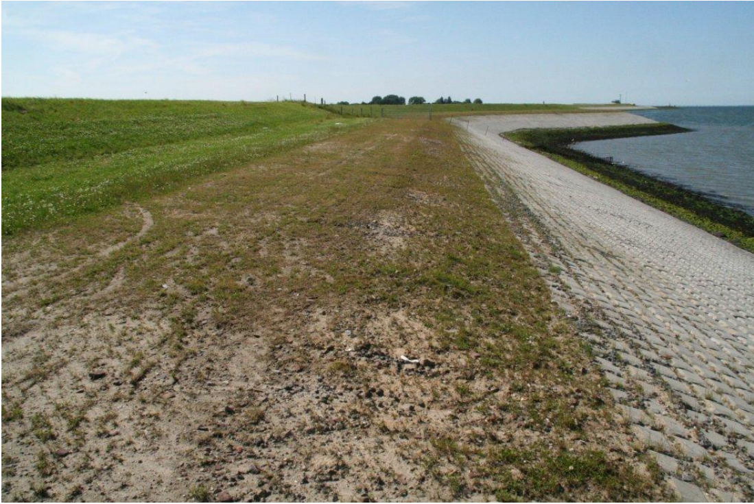
Figure 2.13. Dike near Wemeldinghe, directly after renovation. Design water level 3.6 m +NAP; design wave height 0.9 m.
