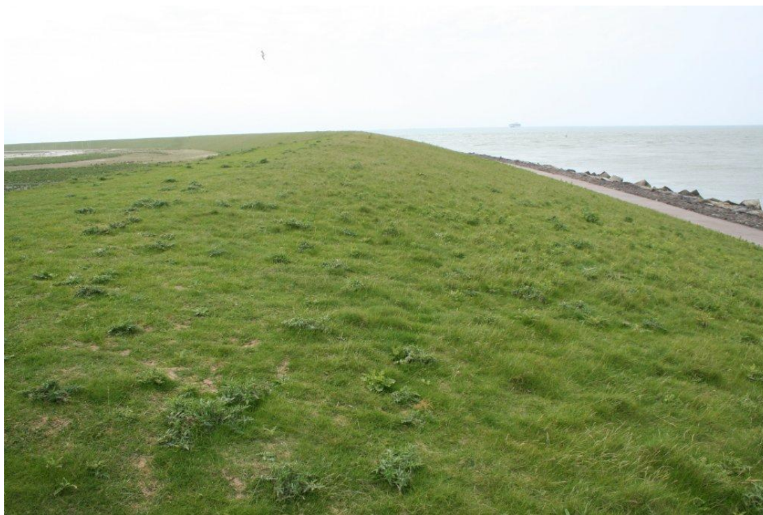
Figure 2.15. Dike at Maasvlakte I, facing the North Sea. Here better grass coverage. Design water level about 5 m +NAP. Design wave height not available, but between 5-8 m.
