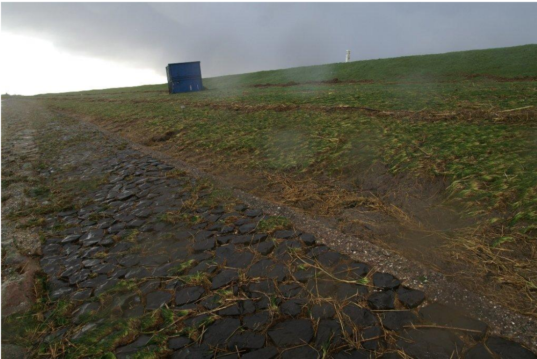
Figure 2.17. Grassed upper slope of a dike at Groningen, damaged by the storm of 1 November 2006.
