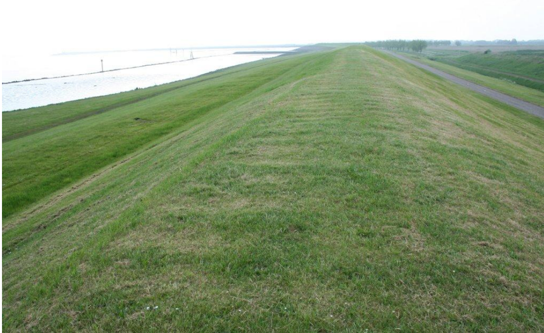
Figure 2.1. Delfzijl - Waddensea. Right side is the landward slope, about 1:3. Left the seaward slope with first a high foreshore, a grassed down slope, a grassed berm and a grassed upper slope. Slopes are about 1:3. This part of the dike is protected for waves to some extent by the breakwaters in front of the harbour.
