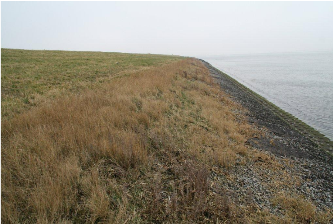
Figure 2.6. St Philipsland - Eastern Scheldt. Seaward side, grassed berm 1:20 with protected down slope 1:3.5.
