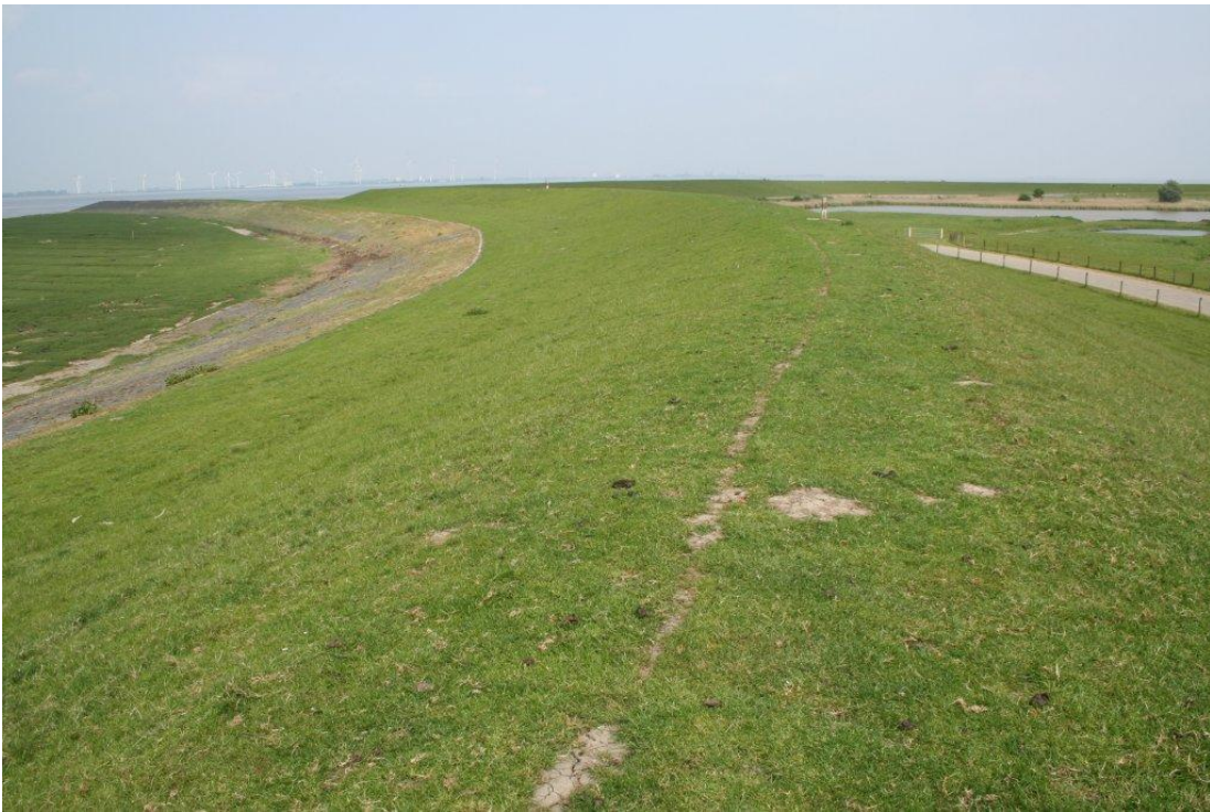
Figure 2.11. Dike Breedbaerdpolder, Groningen. Design water level 6.4 m +NAP; design wave height 1.4 m.
