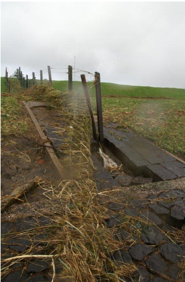
Figure 2.18. Grassed upper slope of a dike at Groningen with a transition. Grass damaged (left side of photo) and transition damaged by the storm of 1 November 2006.
