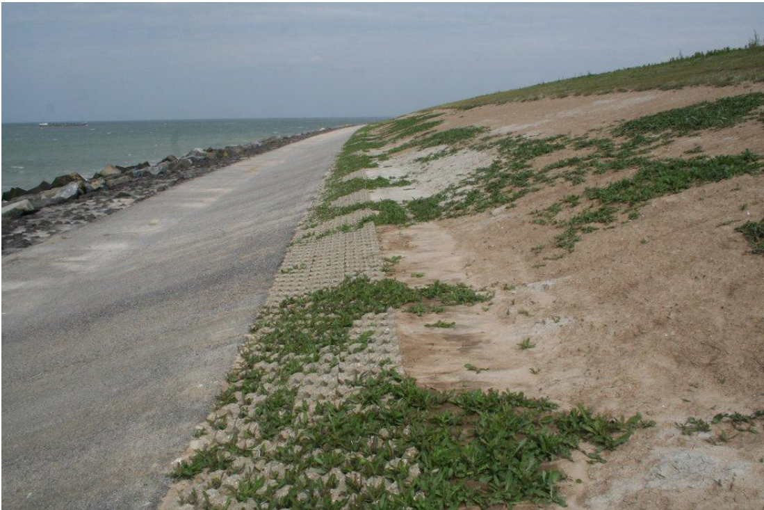
Figure 2.14. Dike at Maasvlakte I, facing the North Sea. At some locations bad grass coverage. Design water level about 5 m +NAP. Design wave height not available, but between 5-8 m.
