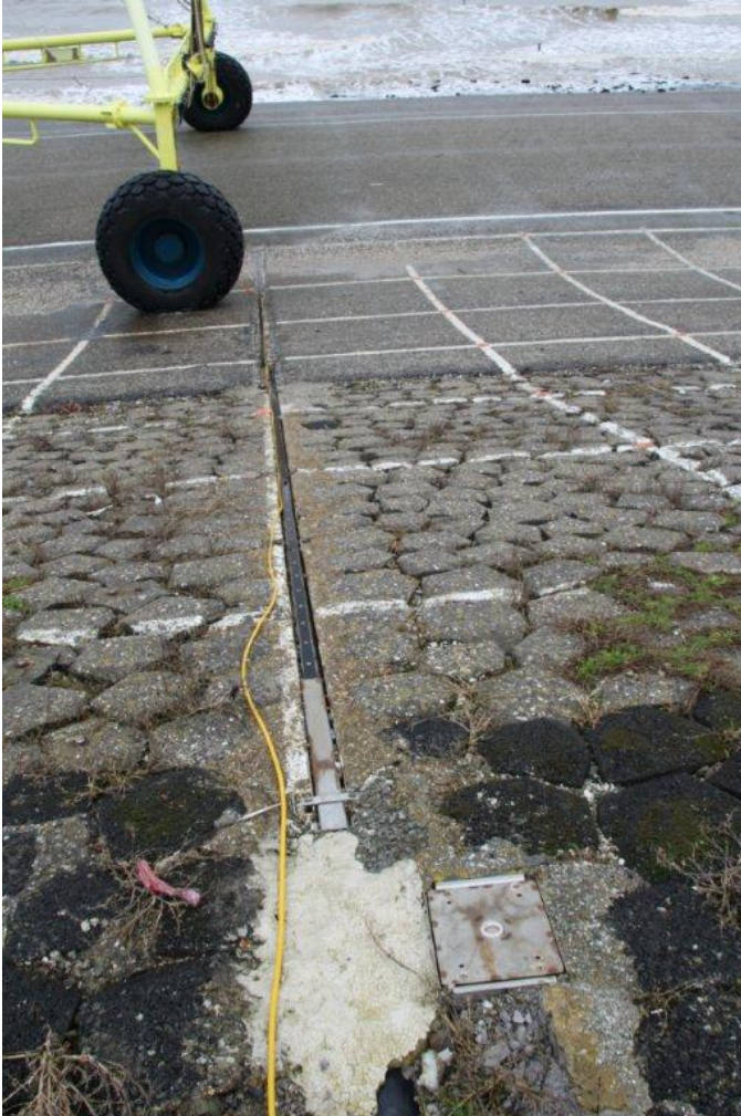
Figure 5.2. Wave run-up gauge at the Petten Seadike, seen from the crest downwards.
