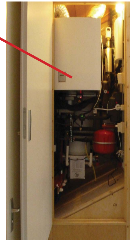
Air ventilation heat pump
