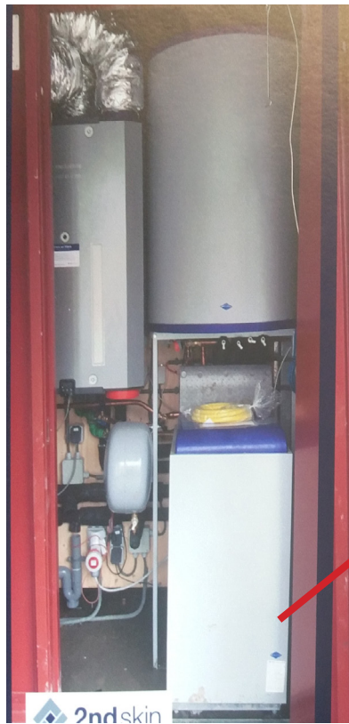
Ground heat pump
