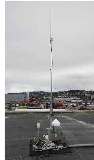
FIGURE 1 The ground station antenna mounted at the top of the array, on the roof of Pirsenteret in Trondheim, Norway.
