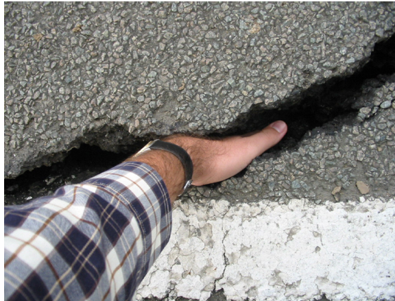
figure A.3-a: crack in asphalt due to transition of foundation
