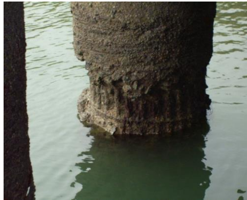
Figure 1-2: Chloride-induced corrosion in a marine environment
