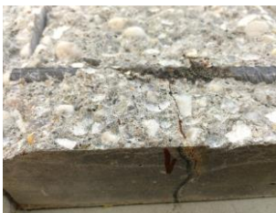
Crack position N°1
