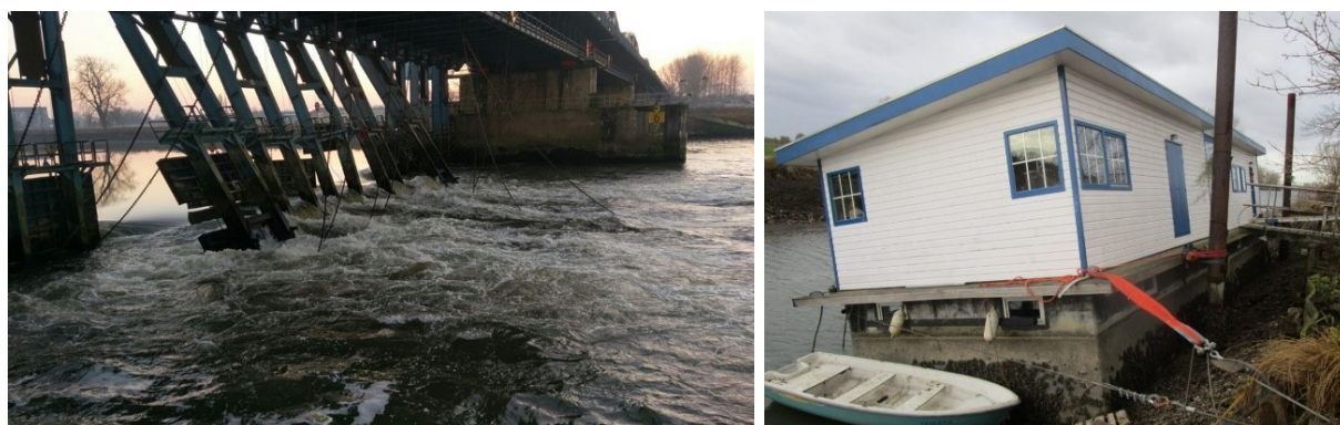
Figure 3.25: Damage to the weir at Grave (left) and the consequences upstream (right) (left: Stuw Grave aanvaring by Nico van Lammeren is licenced under CC0 1.0; right: BootAanBoot.NL , all rights reserved).
