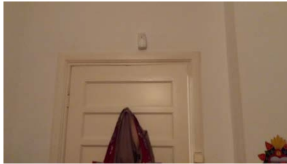
Figure 3.2: PIR sensor mounted above a door
