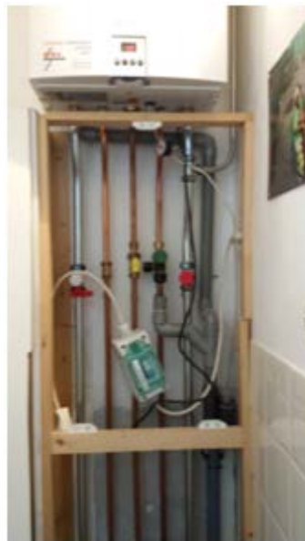
Figure 3.3: Eltako Electricity meter used for measuring in real time the combi-boiler's pump energy consumption
