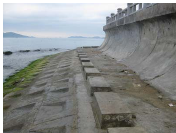
Figure 6.5 Crown wall with wave-deflecting nose and wave-attenuating blocks on the frontal platform
