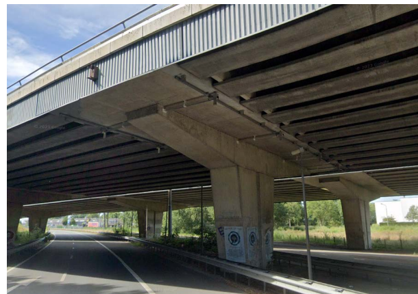
Figure 3: Street view image of support 5 of the southern Naardertrekvaart bridge (Google Maps)
