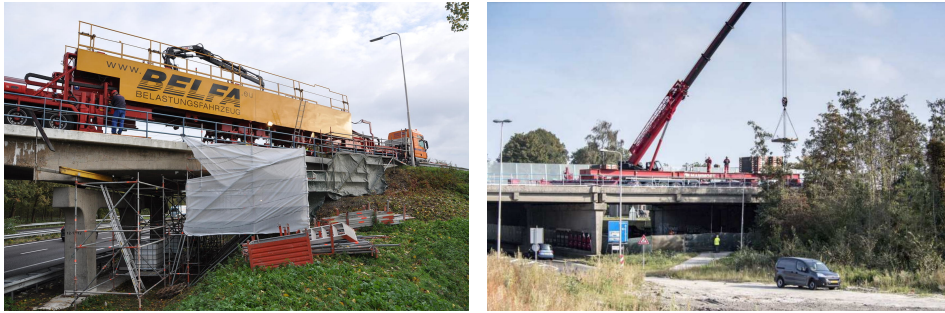
Figure 1.1 Pilot proof load tests in the Netherlands using the specialised BELFA loading vehicle on the Vlijmen-Oost viaduct in 2013 (left) and using a loading frame on the Vechtbrug in 2016 (right). Reprinted with permission from Lantsoght et al. (2017a) and De Vries et al. (2022) .
