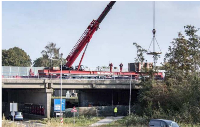
Figure 1. Collapse test being performed in October, 2016 on the Vechtbrug in The Netherlands (De Vries, Lantsoght, Steenberg, & Fennis, 2022).
