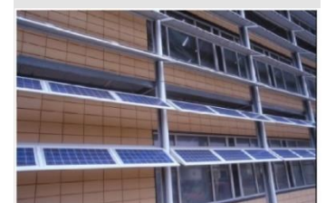
figure 5.2: integrated PV cells in sunscreens with multiple function: shade and produce energy (Kaan & Reijenga, 2002) .
