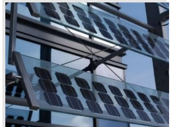
figure 4.18: top: adaptable external shading of tower Al Bahar tower. Middle and bottom: external shading with PV (Wurm, 2007, p. 133)
