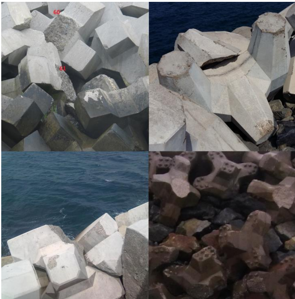
Figure 5.7: Broken concrete armour units, Hofland et al. (2018)
